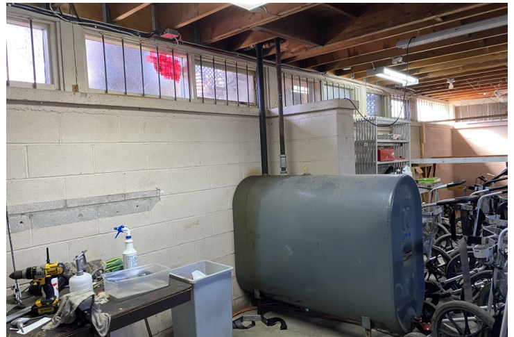
PHOTO 2: View of fuel-oil AST located in the basement of Building B located on the east advanced property.
