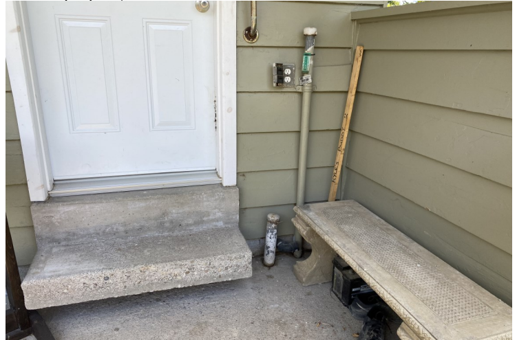
PHOTO 6: View of vent/fill pipes associated with a fuel oil AST at Building D located on the east advanced property.
