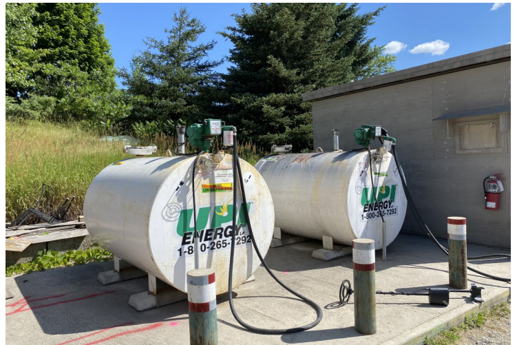
PHOTO 4: View of one (1) diesel and one (1) gasoline AST located adjacent to the east portion of Building C located on the east advanced property.
