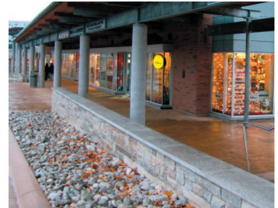
Photo 30: Porous surfaces or landscaped areas should be used to capture roof drainage and minimize water runoff.
