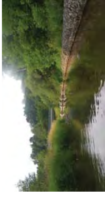
ESMC(1b): Watercourse with undermined gabion baskets
